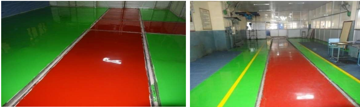
Epoxy Flooring in RB section
